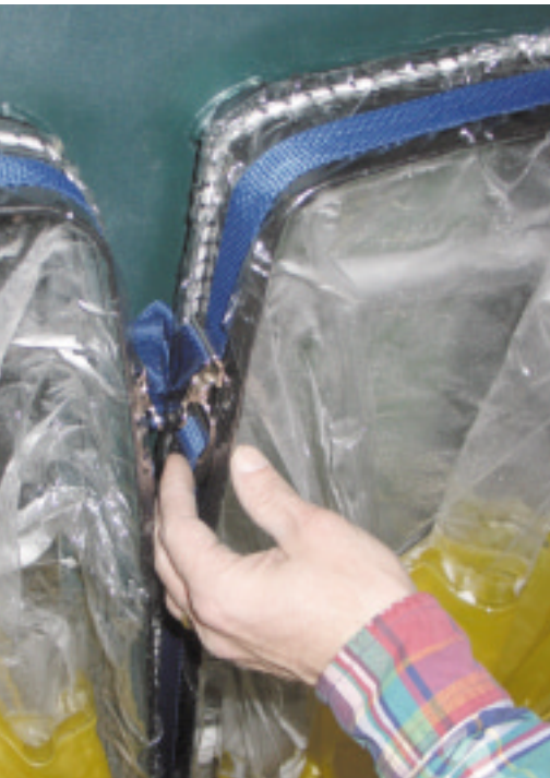
BIBO Filter Access
